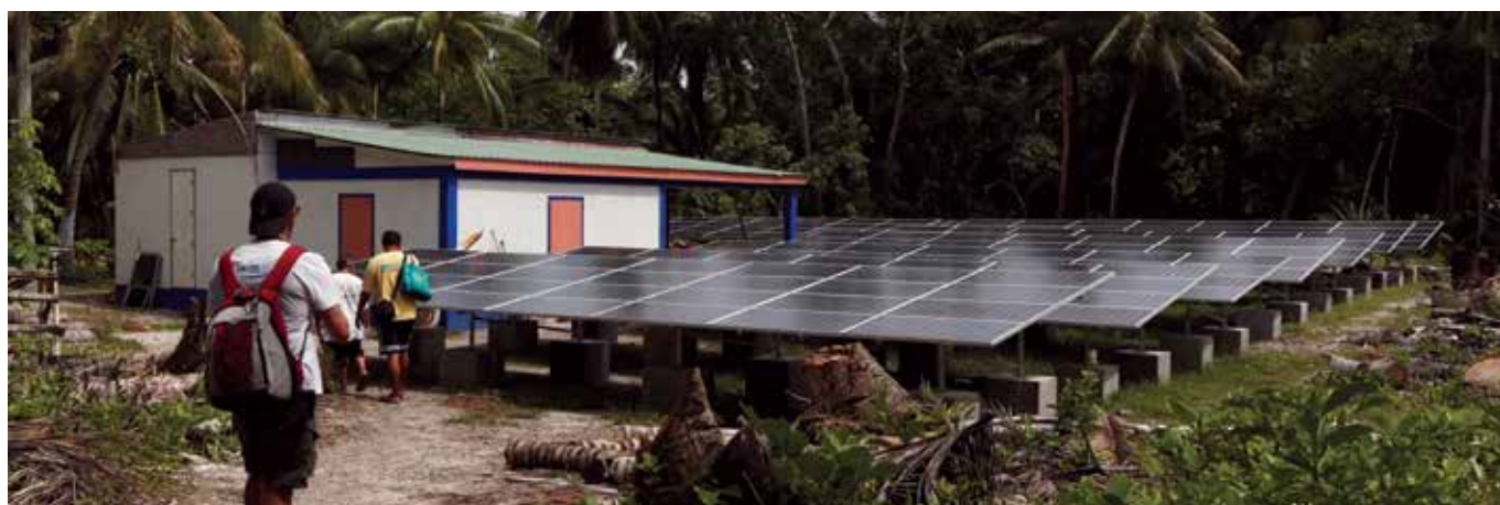
Figure 59: Inspection of a solar mini grid in Mog Mog, Ulithi atoll, Yap State, FSM
