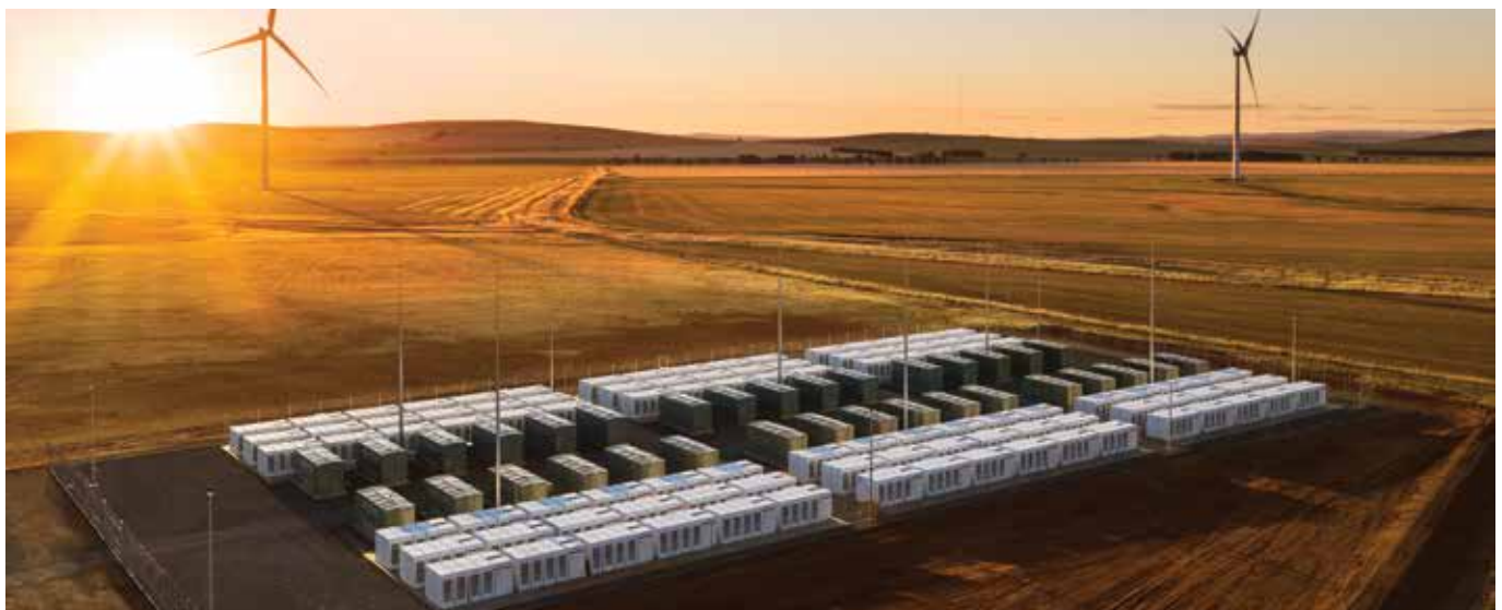
Figure 43: Hornsdale Power Reserve in South Australia
