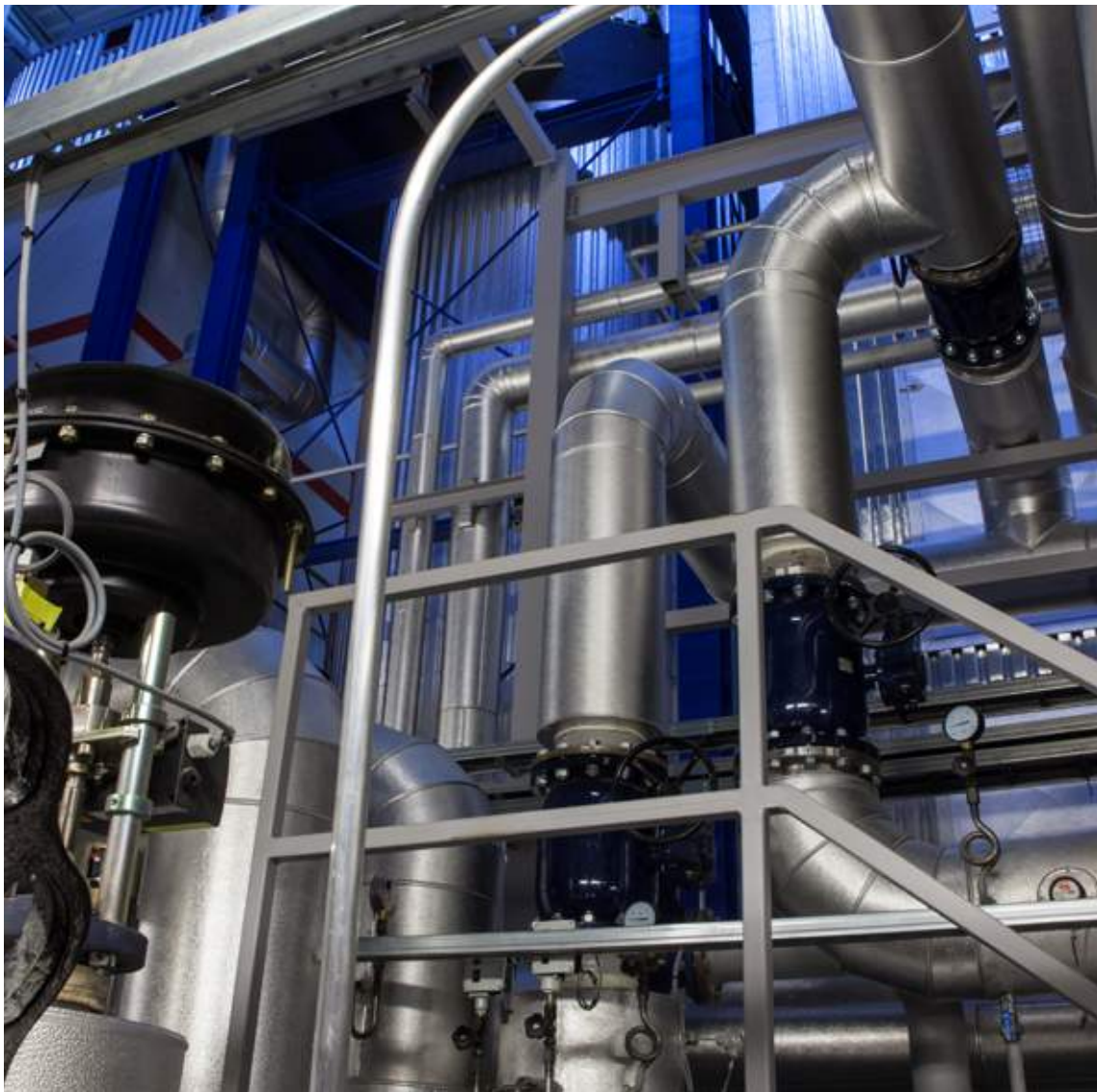
Modern biomass co-generation power plant.
