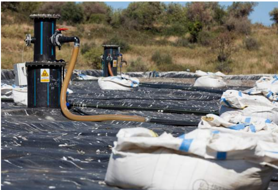
Landfill captured biomethane in Italy.
