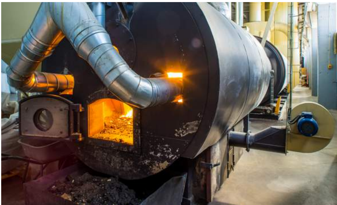
Wooden pellets boiler.
