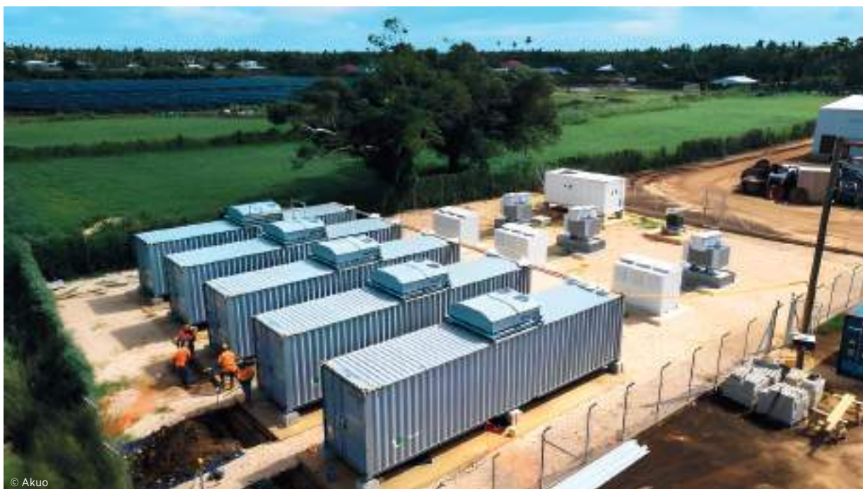
Figure 6 Tonga's Battery Storage
