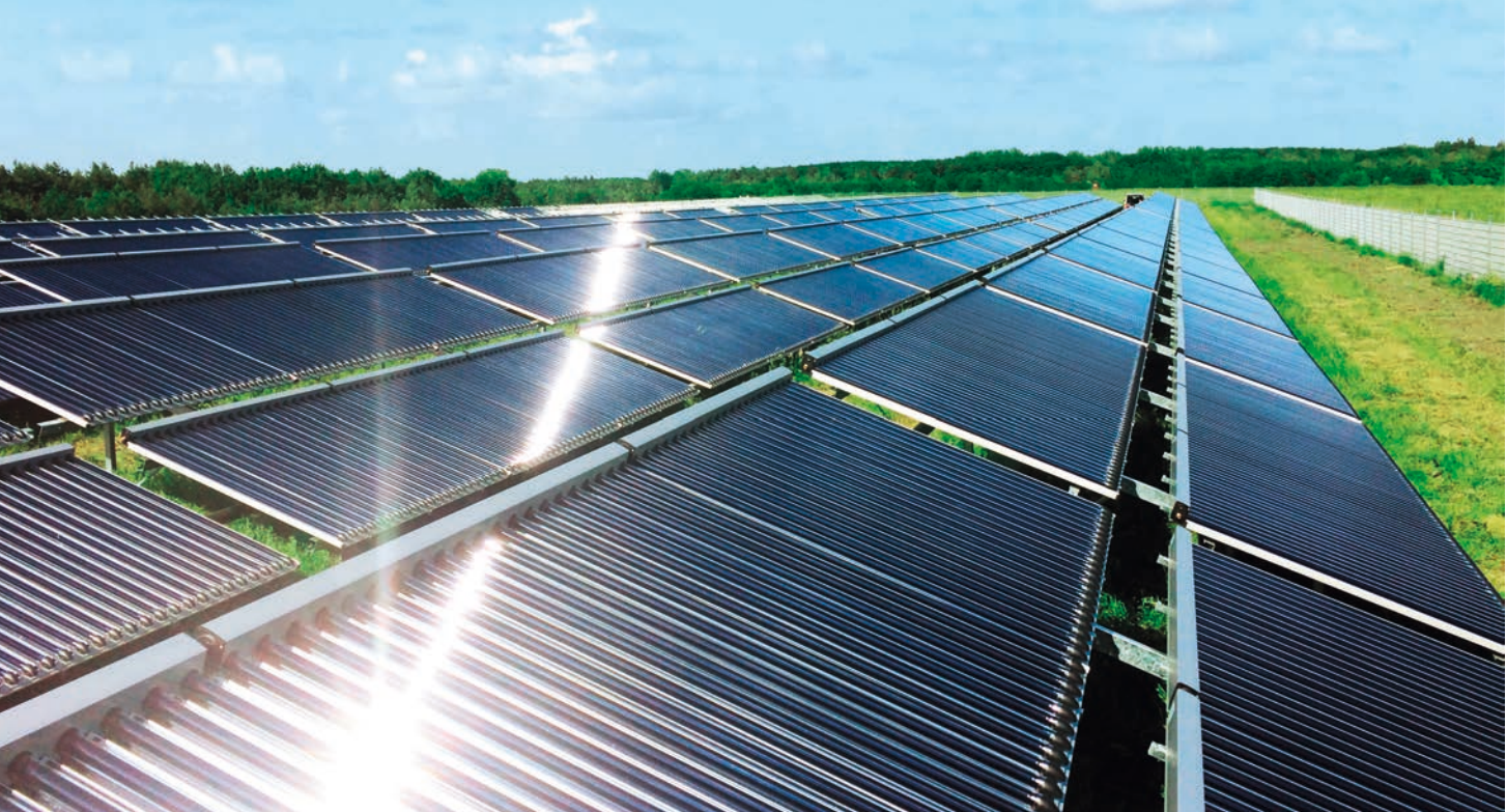
Solar District heating system with 18,732 m 2 evacuated tube collectors in Greifswald, Germany Photo: Ritter XL Solar
