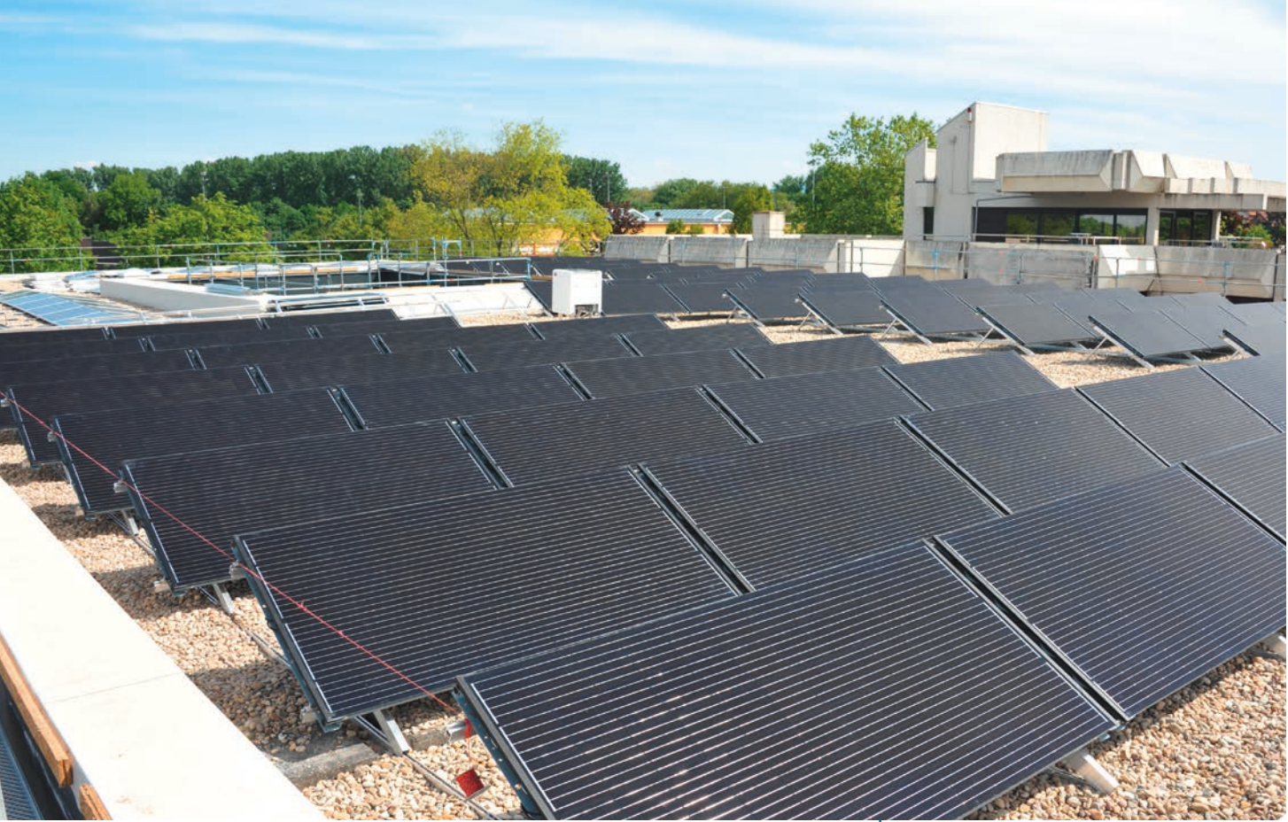
200 m 2 PVT-collector field for a new office/council building in Offenbach an der Quaich, Germany Photo: Consolar, Germany
