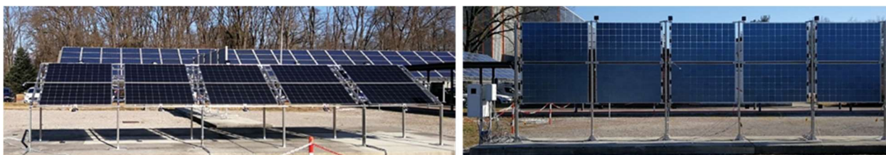
Figure 11. ESTI outdoor test field installation of bifacial racks: South-oriented tilted equator facing bifacial solar tracking systems (left) and fixed- vertical bifacial PV module array East-West oriented (right).
