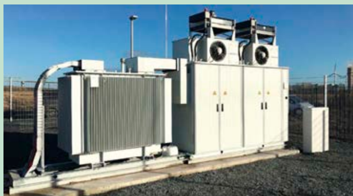
Figure: Battery storage power plant, Wind to Gas Energy Photo: Wind to Gas Energy GmbH & Co. KG 32
